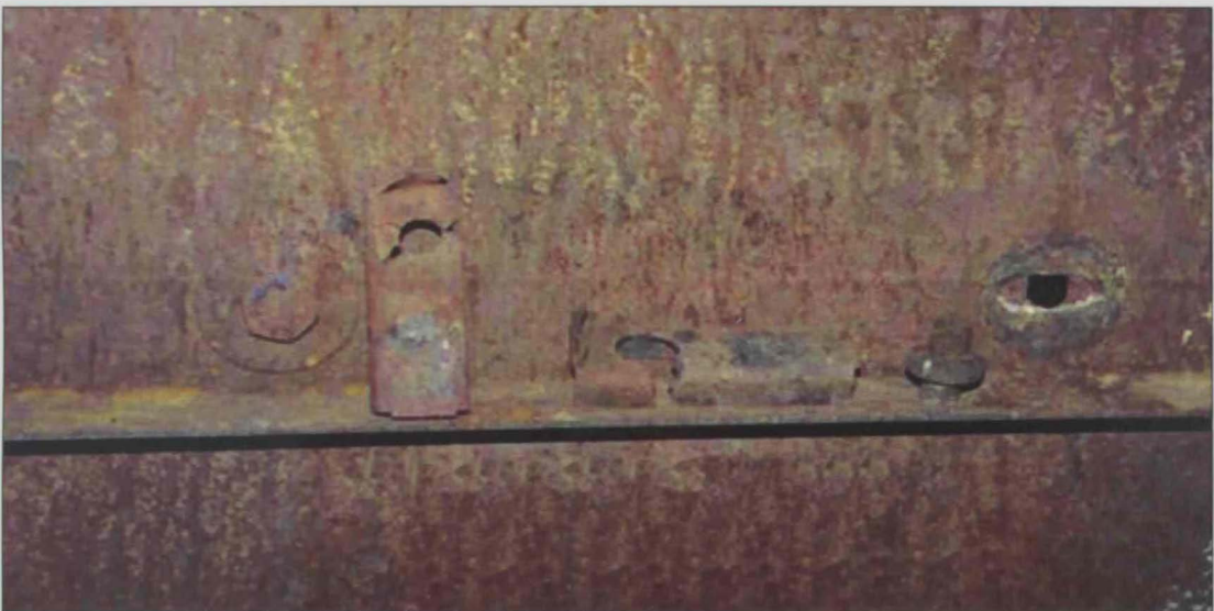
Figure 5: Corroded stainless steel clip and its location inside condensate stabilizer
