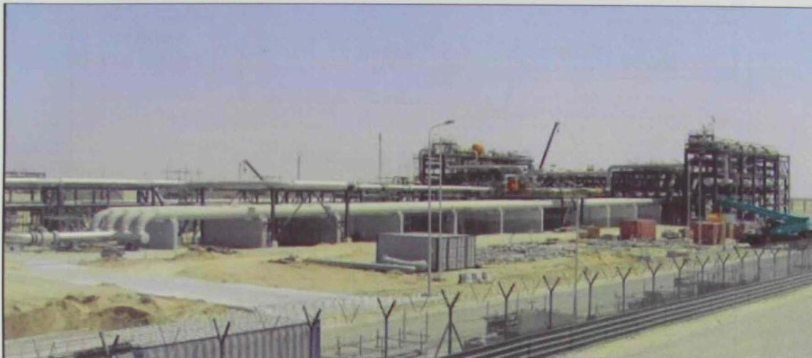
Figure 12: Slug Catcher at the condensate recovery plant battery limit
